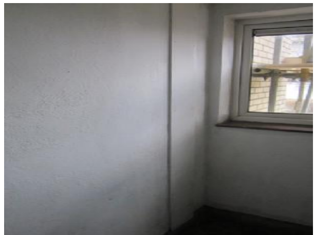
AIB risers in communal areas
