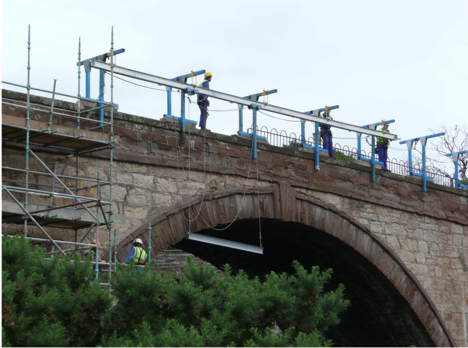
ADT Installation; 4 ALPS operatives taking 1-1/2 days to install 60M of track at road level
