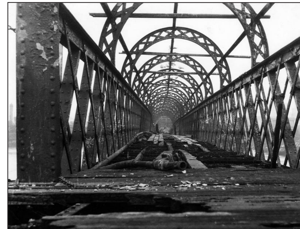
The war-damaged pier – note the blistered paint and the burnt and buckled timbers of the walkway.
