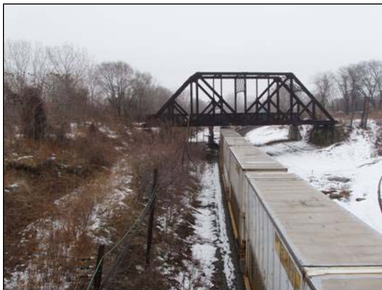
Photo 167: Olive Secondary Track Bridge over the NS Cleveland-Chicago Mainline MP 287.5 – View east
