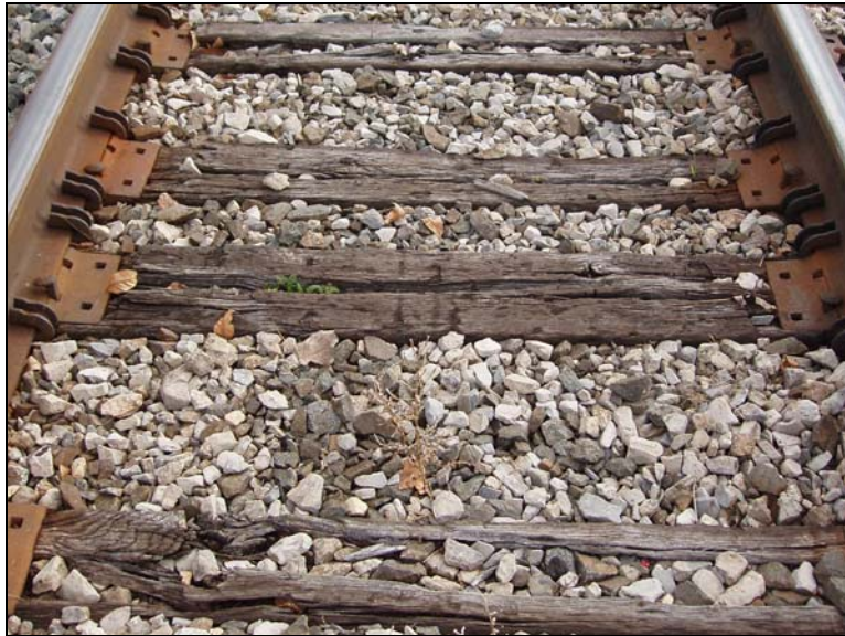
Photo 120: Fort Wayne Line at Peterson Rd, east of Ada at MP 242.6 - Close up of Rotted Tie Conditions
