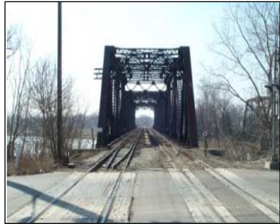
Photo 17: Looking north at CN MP 17.7, double track bridge over the River Raisin in Monroe
