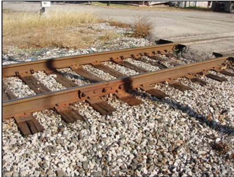
Photo 132: Fort Wayne Line, Mason St grade crossing MP 280.3 in Middlepoint – Close up
