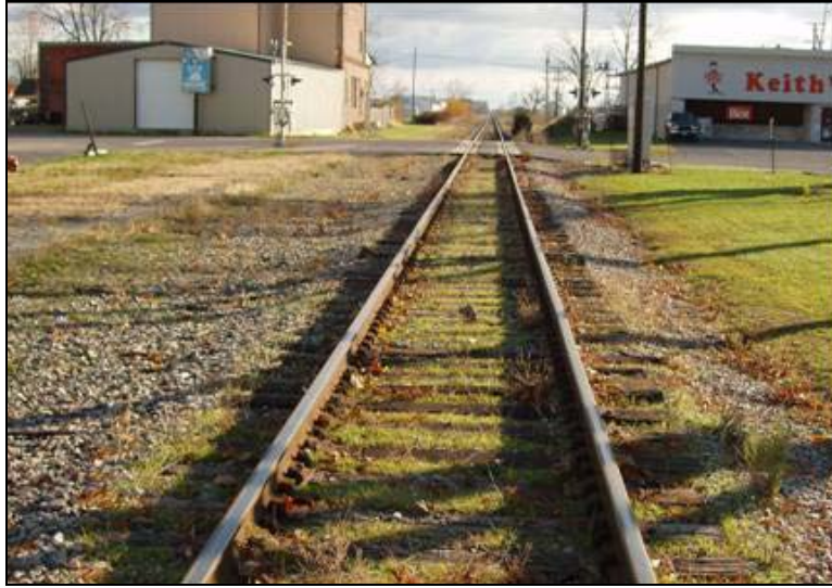
Photo 122: Fort Wayne Line at Ada historic passenger station MP 245.5 - View east – Another view of the track in front of the station
