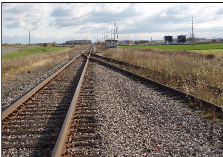
Photo 119: Fort Wayne Line at Peterson Rd, east of Ada at MP 242.6 - View east
