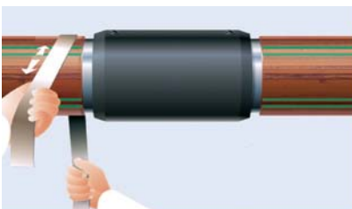
Fig 8-25: Sanding the protective coating in the region of the heat shrink sleeves
