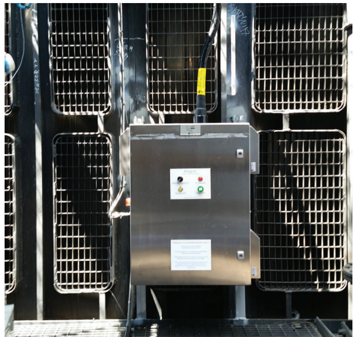
Emsys enclosure installed on the weather deck close to scrubber outlet
