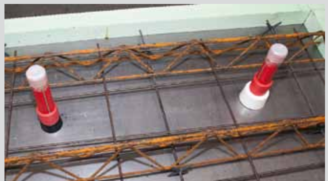
1. Type of connection: visible sprinkler
