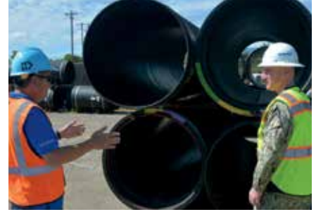
Hawaiian Dredging Construction Co. Inc. broke ground in August on NAVFAC’s $48 million P-169 Water Transmission Line at Joint Base Pearl Harbor-Hickam.
