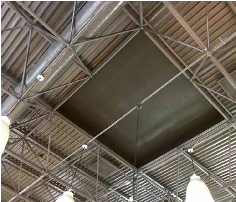
New soffits and dropped ceilings, designed by AHL and installed by THG, open up JP Superstore’s interiors. PHOTO COURTESY TUTUJAN HILL GROUP LTD.
