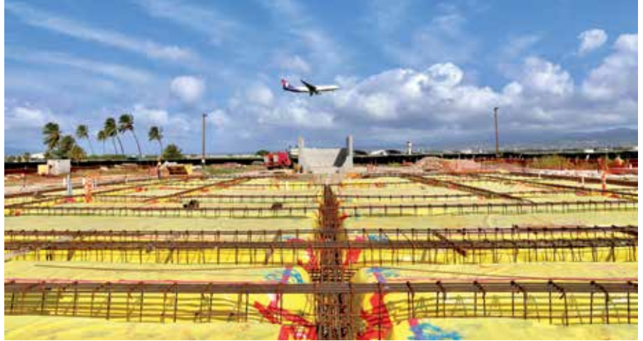
Nordic PCL's foundation work at the F-22 Fighter Alert Facility PHOTO COURTESY NORDIC PCL CONSTRUCTION INC.
