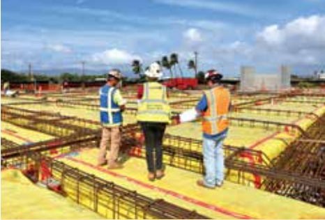
The Nordic PCL team uses a proprietary program at the F-22 Fighter Alert Facility. PHOTO COURTESY NORDIC PCL CONSTRUCTION INC.
