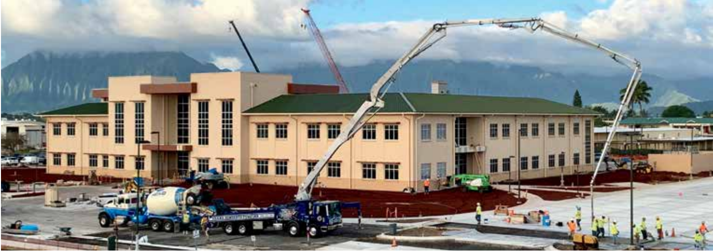
Cadell-Nan Joint Venture installs a parking area next to a new, two-story, 96,000-square-foot-plus structure that will consolidate all medical and dental facilities on Marine Corps Base Hawaii. The $82.6 million project, shown here in late 2019, will wrap in December 2020.
