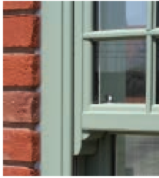
Run through sash horns
