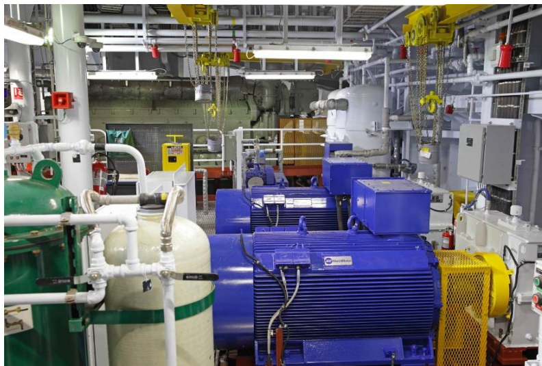
Jet Pump Motors - Engine Room
