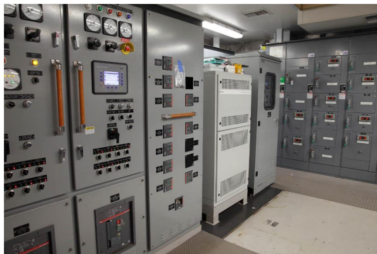
Dredge Switchgear Room
