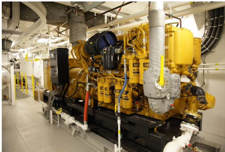
730kW Caterpillar Auxiliary Generator
