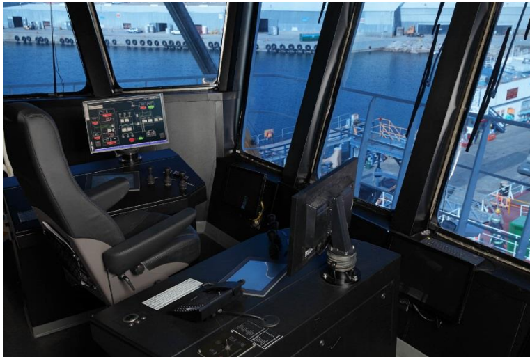
Dredge Control Station
