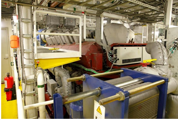
MAK Diesel Main Engine
