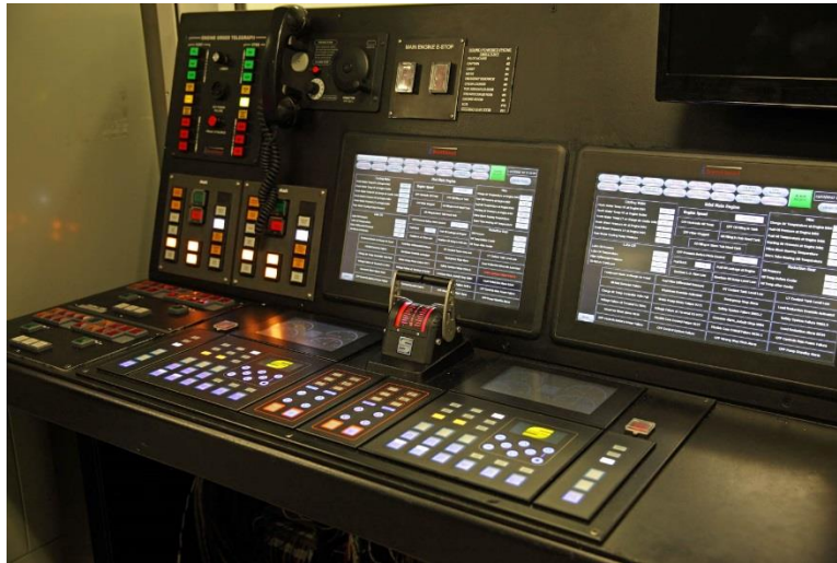
Engine Control Room
