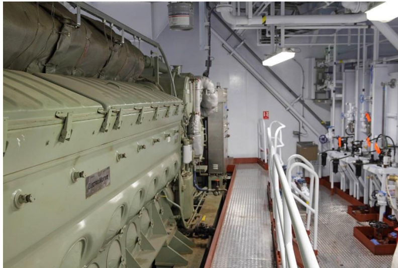
Dredge Pump 5,000HP EMD Diesel Engine
