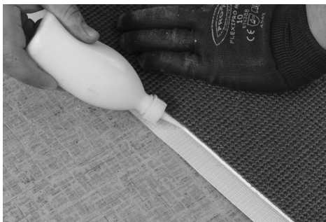
Adhesive for seams very sparingly in a linear manner along a lath
