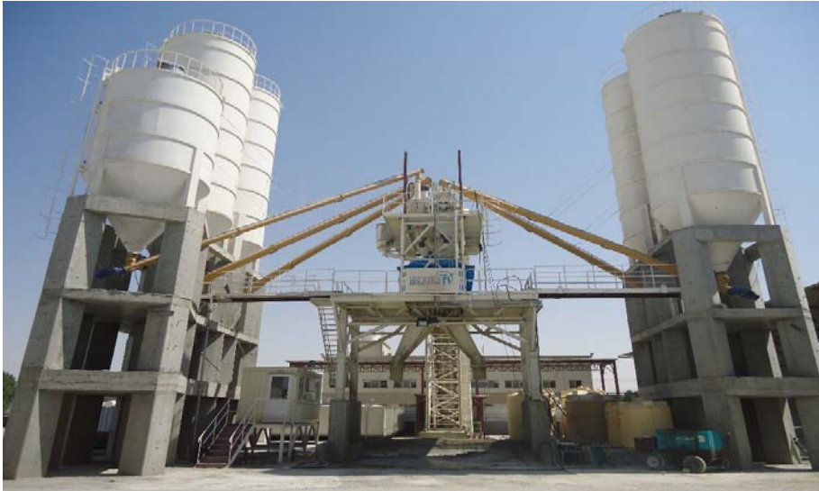
CONCRETE BATCH PLANT
