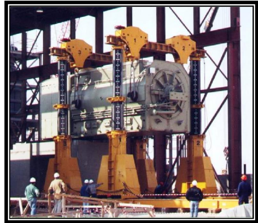
J&R 1402-4-39 Octagon LIFT-N-LOCK Hydraulic Boom Gantry with 150 Ton PowerLinks on a project in Riyadh, Saudi Arabia
